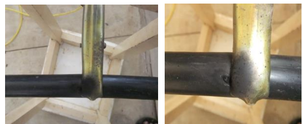
Figure 5. Failure of XLPE cables
